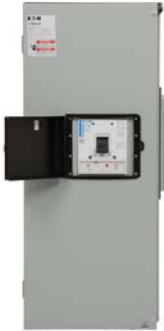
Main Circuit Breaker
