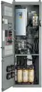
Enclosed 18-Pulse Drive
